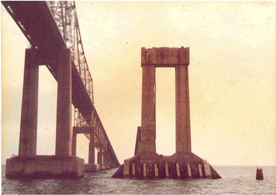
Another photo of Pier 1-S showing its counterpart holding up the northbound span, also taken in 1981. The space between the two piers is where the southbound span fell into after impact by the Summit Venture. The two piers are different as the pier to the right was the one repaired in 1969 due to settling and cracks which required pilings driven deeper below the water surface until limestone was reached.
